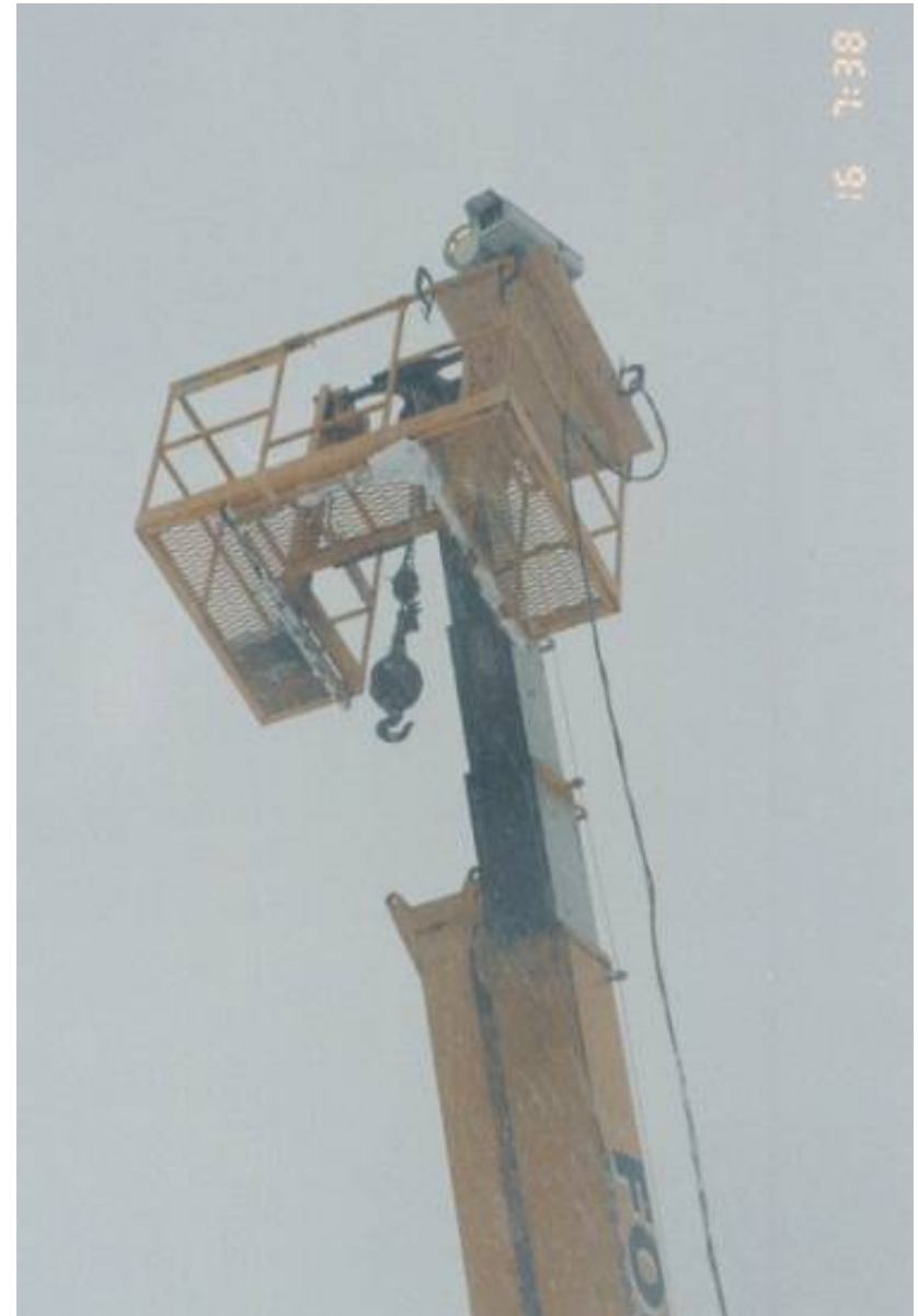
Photo 2.2 Sensor Installation on Bucket
