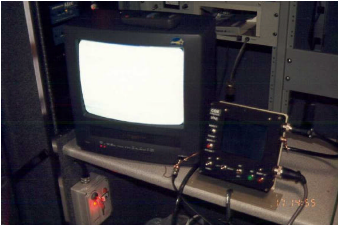
Photo 2.17 Ice Detection Camera Monitor and VCR in Cabin
