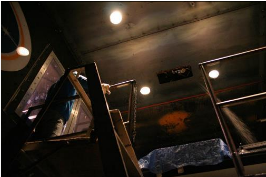
Photo 2.8: Ceiling Mounted Freezing Rain Sprayer
