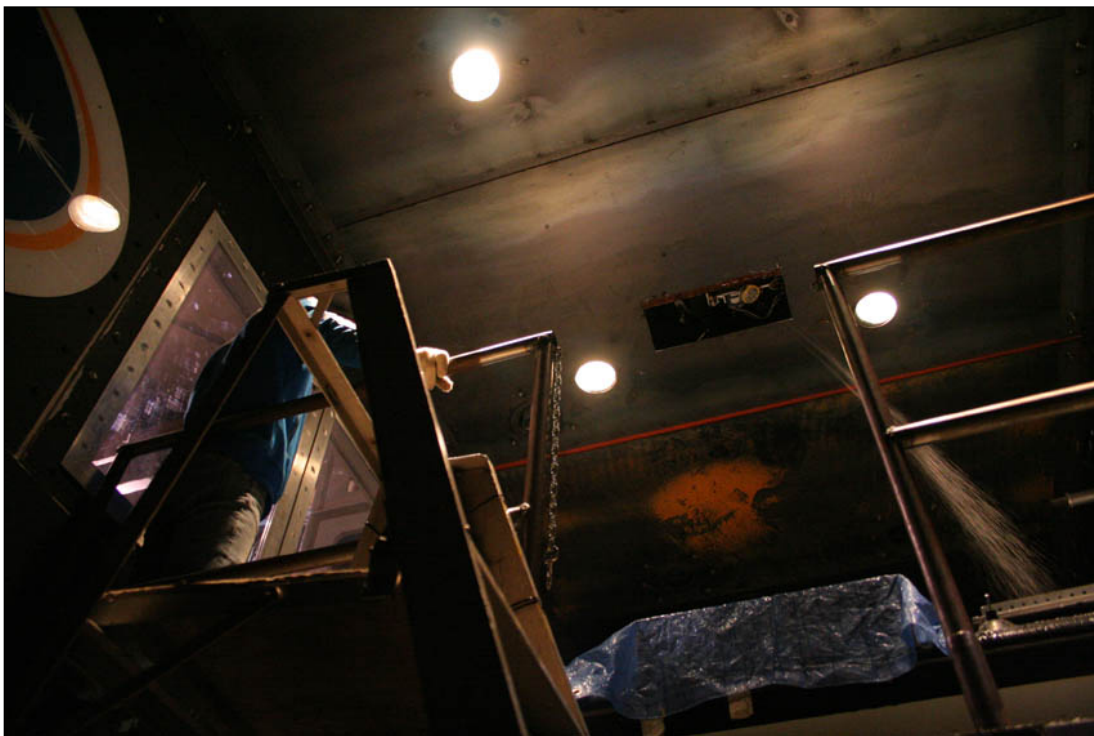
Photo 2.8: Ceiling-Mounted Freezing Rain Sprayer
