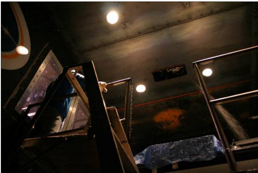
Photo 2.8: Ceiling-Mounted Freezing Rain Sprayer
