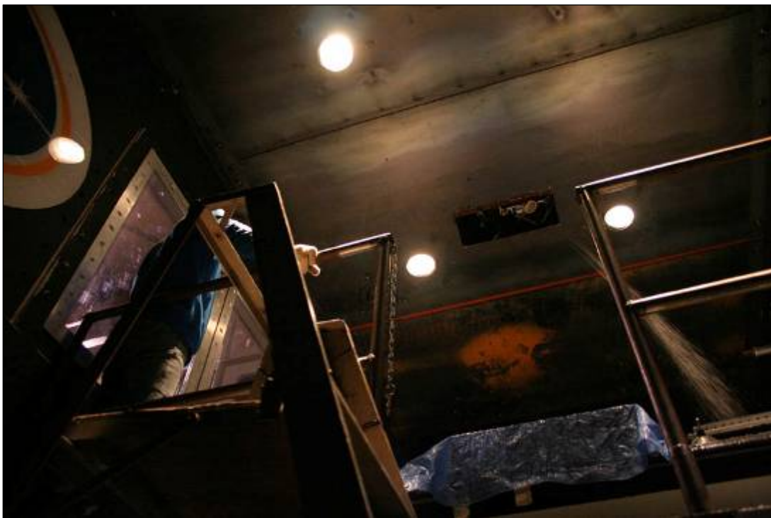
Photo 2.8: Ceiling-Mounted Freezing Rain Sprayer
