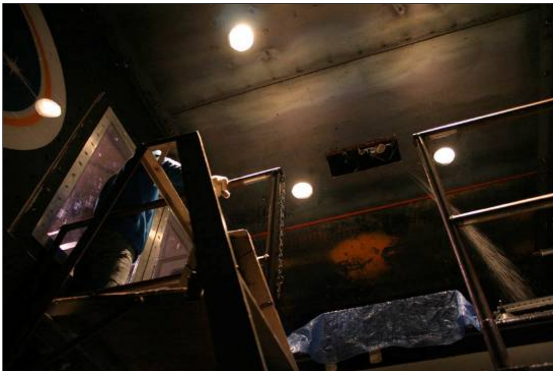
Photo 2.8: Ceiling-Mounted Freezing Rain Sprayer
