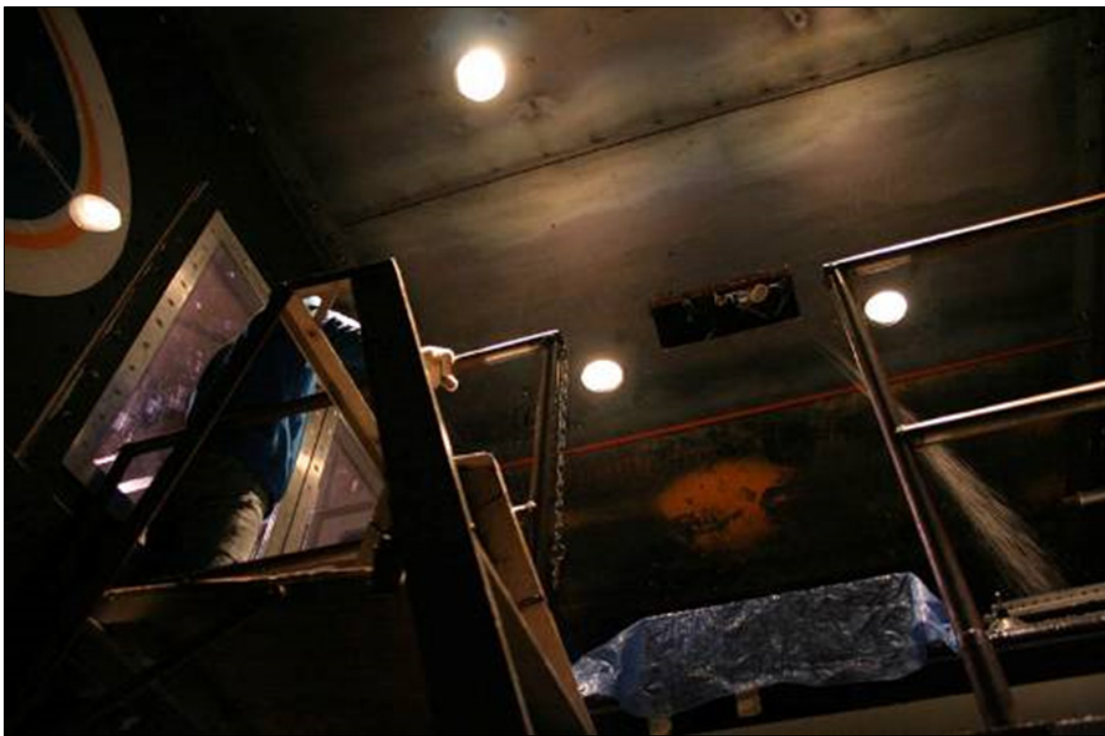
Photo 2.8: Ceiling-Mounted Freezing Rain Sprayer
