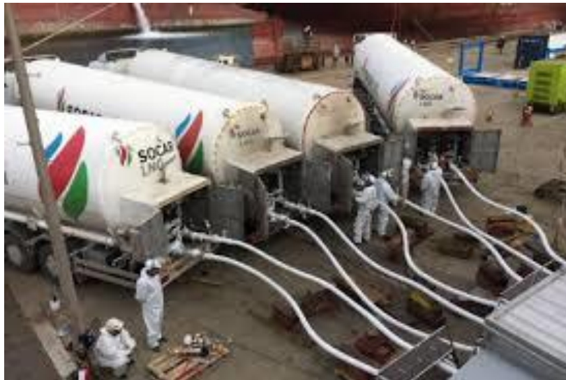
Figure 24: truck Bunkering Manifold System
