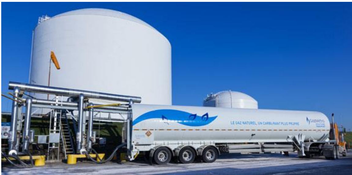
Figure 90: Énergir LNG loading facility in Montréal East, Que.
