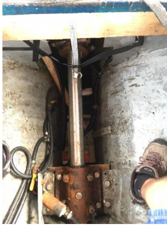
Figure A - 46 Hardware installation on tour boat
