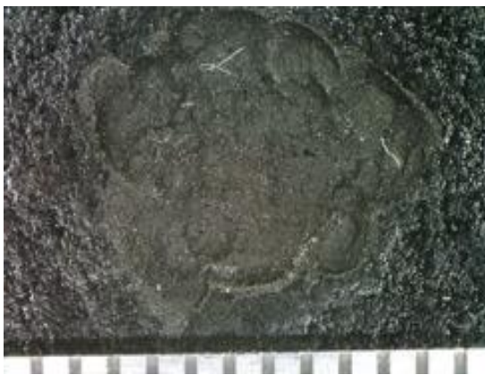
Figure 2-24: Evo2 on 7660 - Observed damage after 10 s at 1.25” offset, 45 deg.
