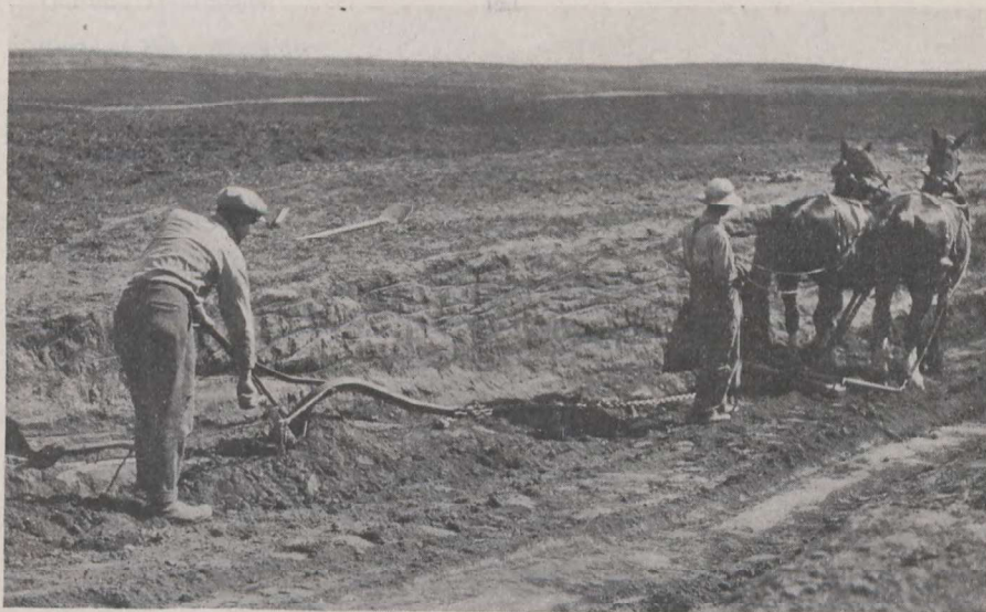
Excavating for a trench silo. A chain is used on the plough in order to keep the walls perpendicular.
