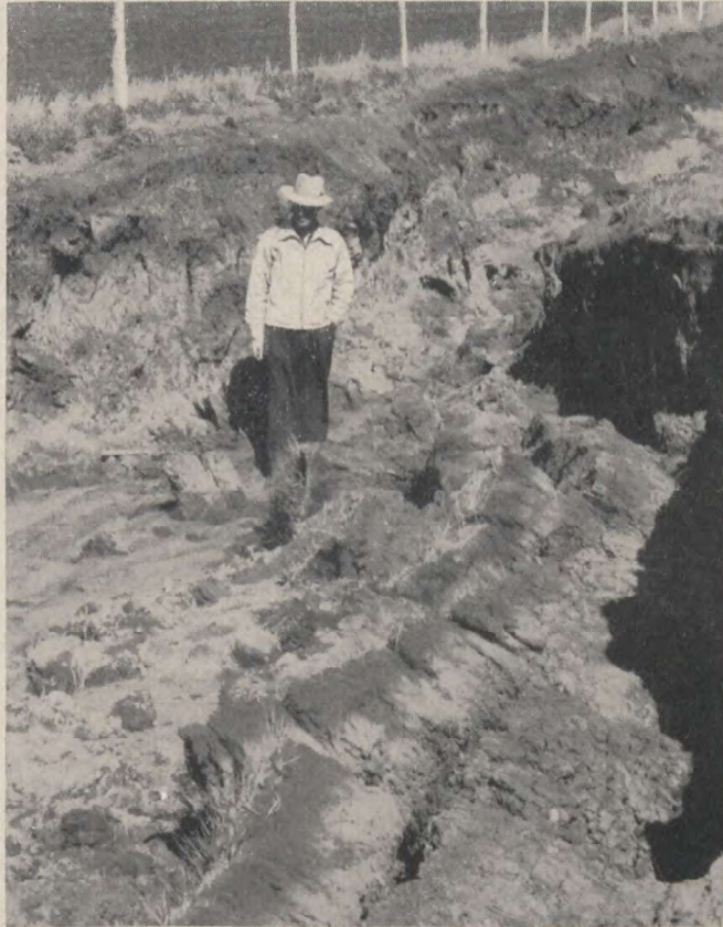
FIG. 4.—Severe gulying resulting from heavy flow of water in an inadequate V-ditch.
