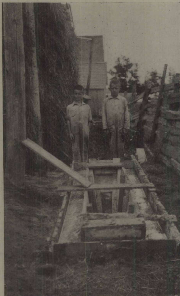
Concrete sheep dipping tank under construction on the Illustration Station at St. Peters, P.E.I.
