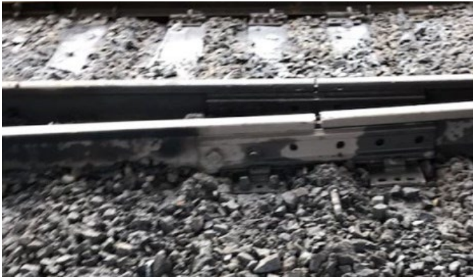
Figure 4. Pull-apart at Mile 116.67 (Source: Canadian Pacific)
