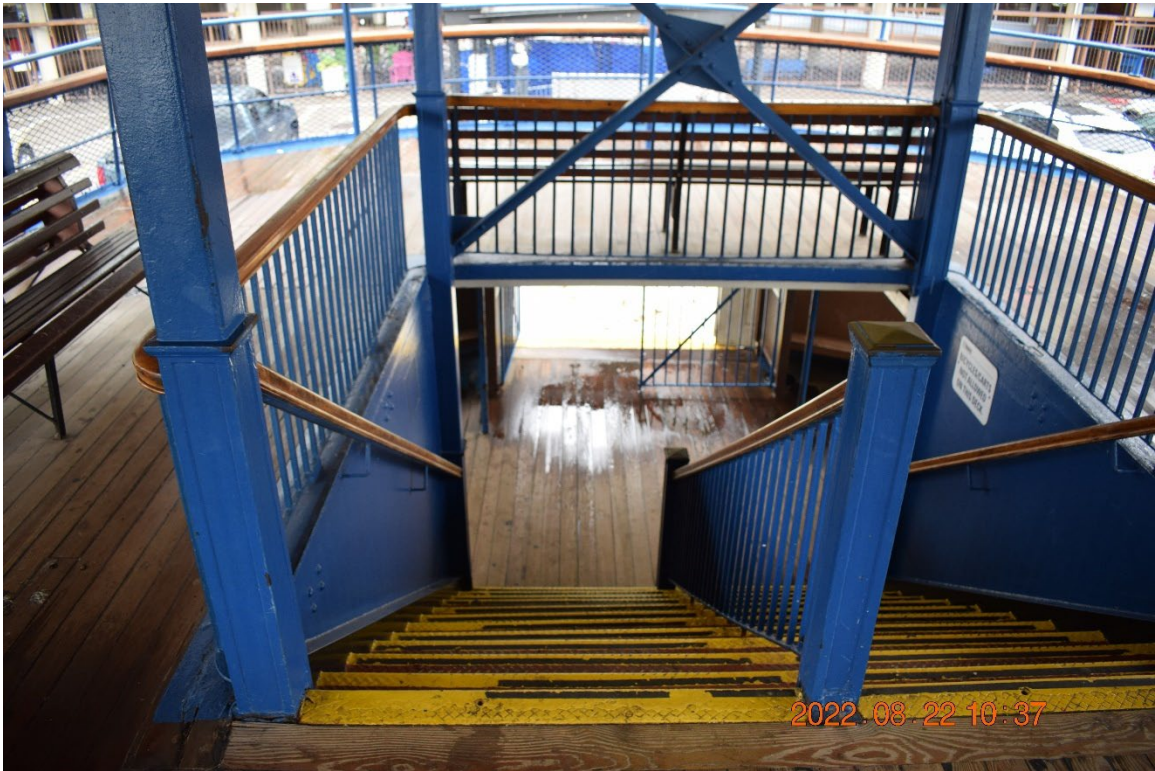
Figure 3. Stairs descending from the promenade deck to the main deck (Source: TSB)
