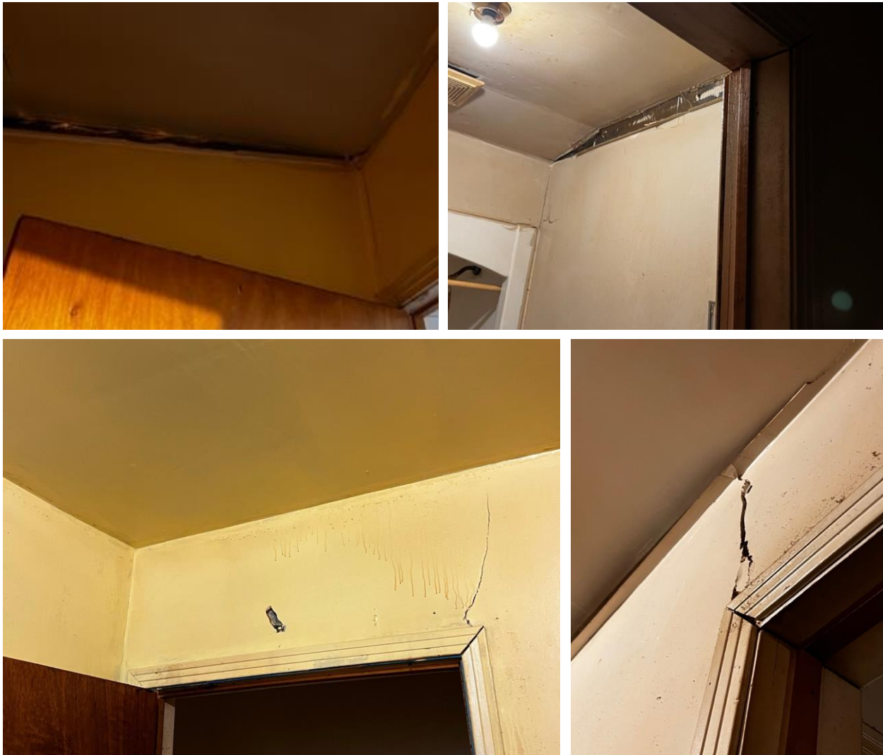
Homes with mould and cracks due to shifting.
