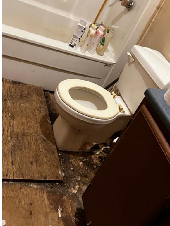
Running toilets lead to condensation on the outside of the bowl, which over time, compromises the integrity of the subfloor around the toilet and creates mould.
