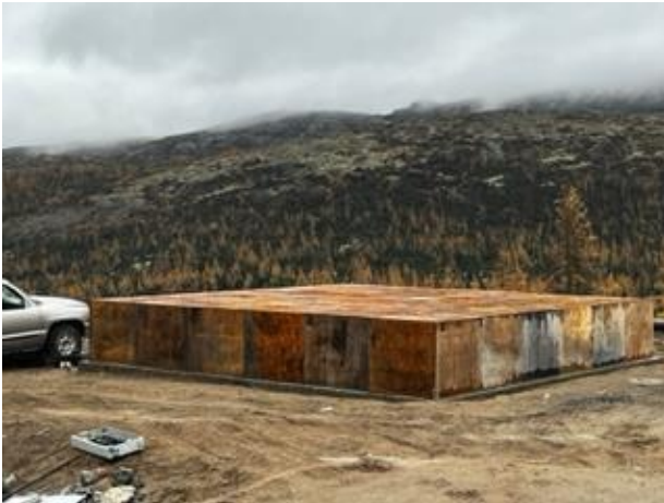
Despite evidence of failures of exposed wood foundations, the practice is still continued for new foundation.
