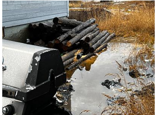
Water collects around a house that has not been graded to allow for adequate drainage.
