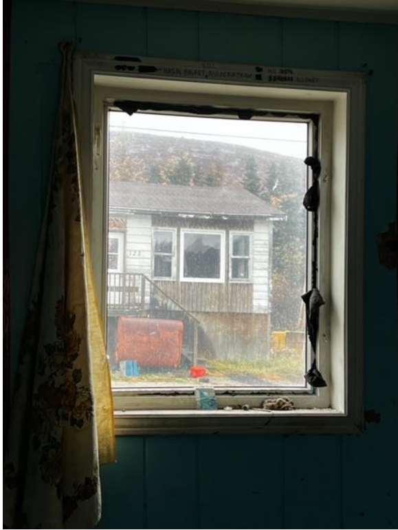
Improperly sealed windows.
