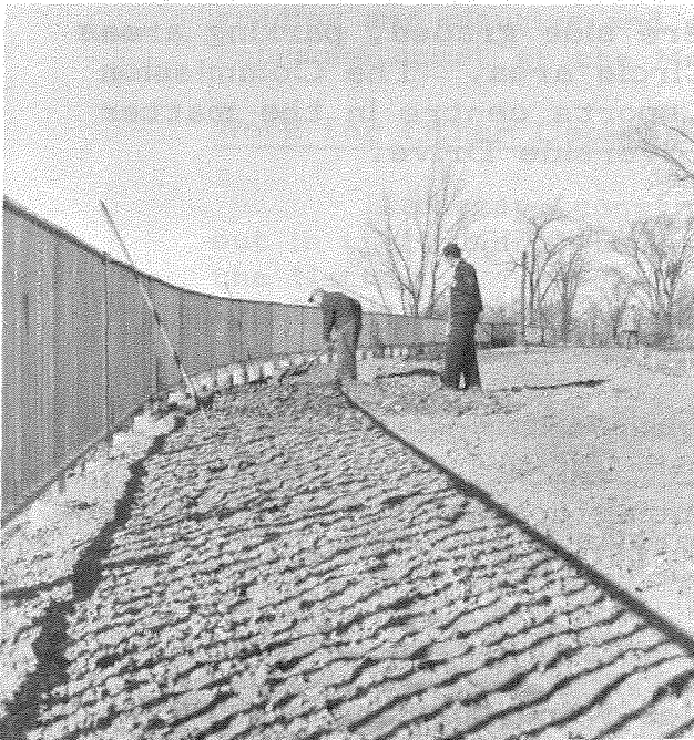
Major's Hill Park - As part of NCC Winter Works program, a new wrought iron fence was built along the bluff. Paths were remade and new flower beds added in the Park.
