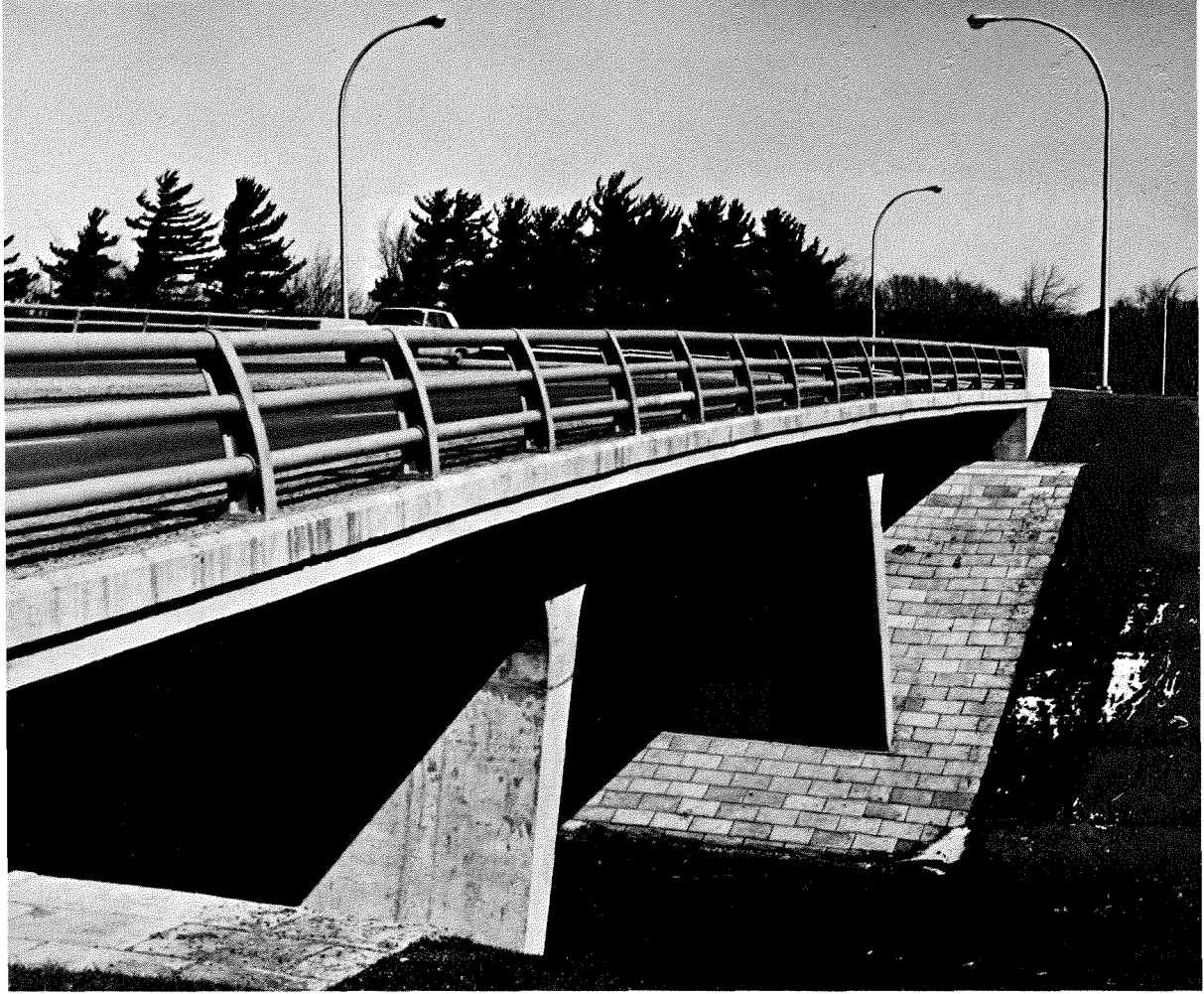
Riverside Drive overpass crossing the CPR Prescott Sub- division tracks in the vicinity of Confederation Heights.
