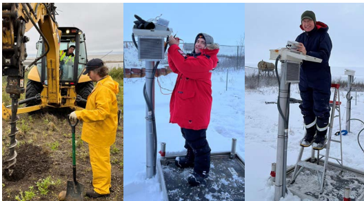
National Research Council of Canada's Dennis Krysz, Antal Prigli and Igor Egorov (from left to right), and their partners are assessing various permafrost mitigation techniques and their effectiveness in combating permafrost thaw.
