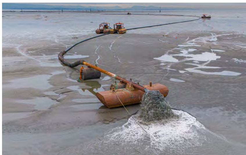
A temporary pipeline deposits reclaimed sediment dredged from the Fraser River onto Richmond's Sturgeon Bank, which is experiencing recession and is threatened by the impacts of rising sea levels.
