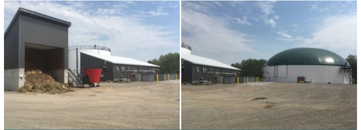
Biogas plant at the Toronto Zoo that turns animal feces and inedible food waste into renewable power for the Ontario grid (photo credit: Zooshare Biogas LP)
