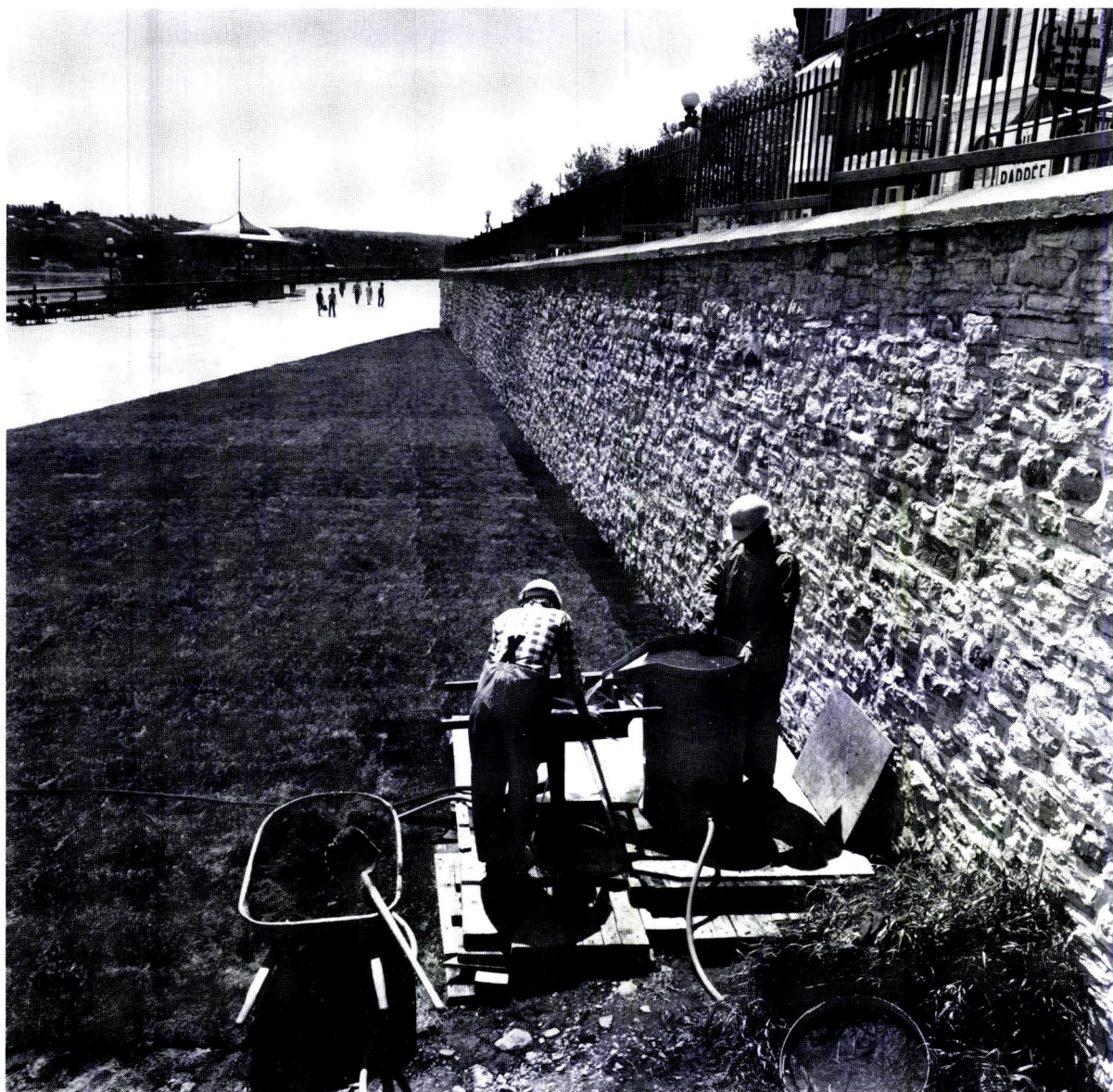
7.2 View of the Dufferin Terrace and the flotation apparatus.
