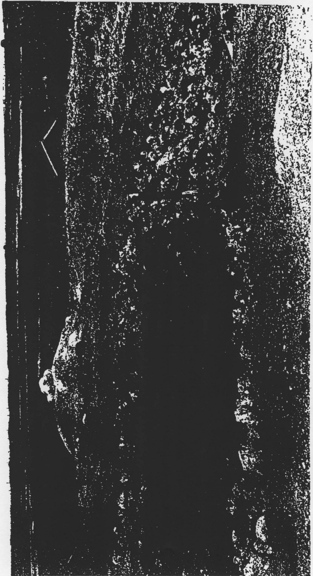
Photograph 3 Poorly maintained road.
