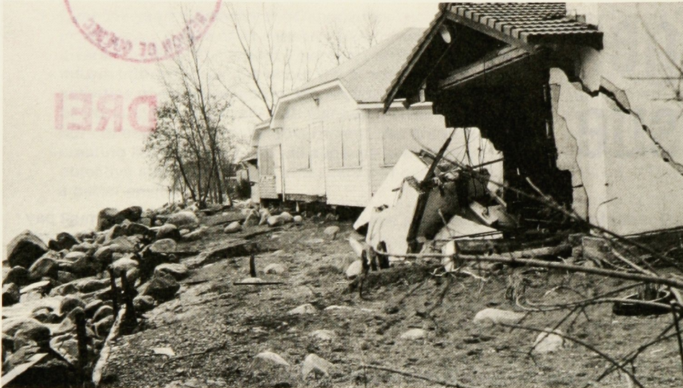
When persistently high supplies to a water body affect the level, widely-spread damage to shoreline property can occur.
