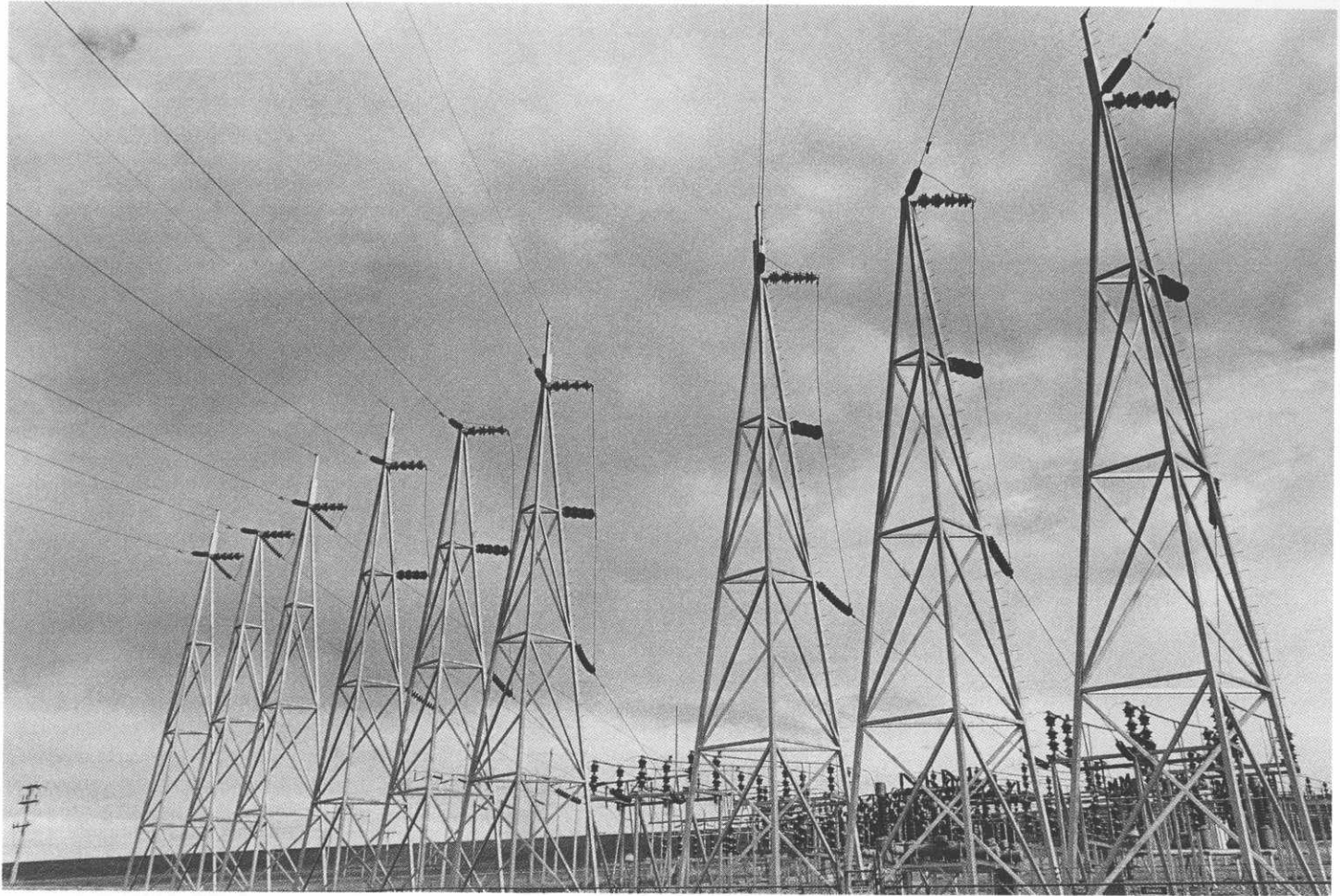
The Coteau Creek Generating Station produces about one million megawatt-hours of electricity each year
