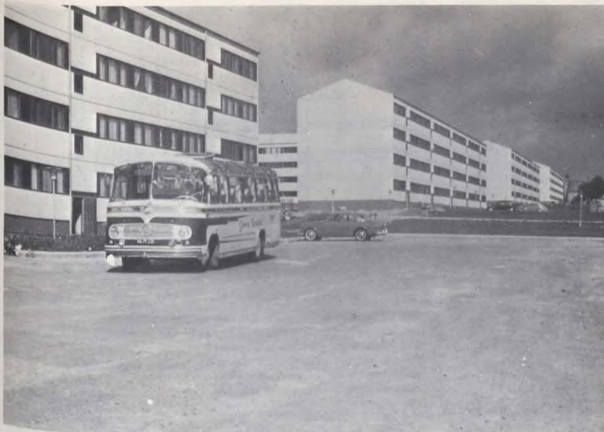
Construction site near Copenhagen. Façade panels are wood framed with sliding windows, the exterior face is of asbestos cement sheets and the interior face of gypsum wallboard.
