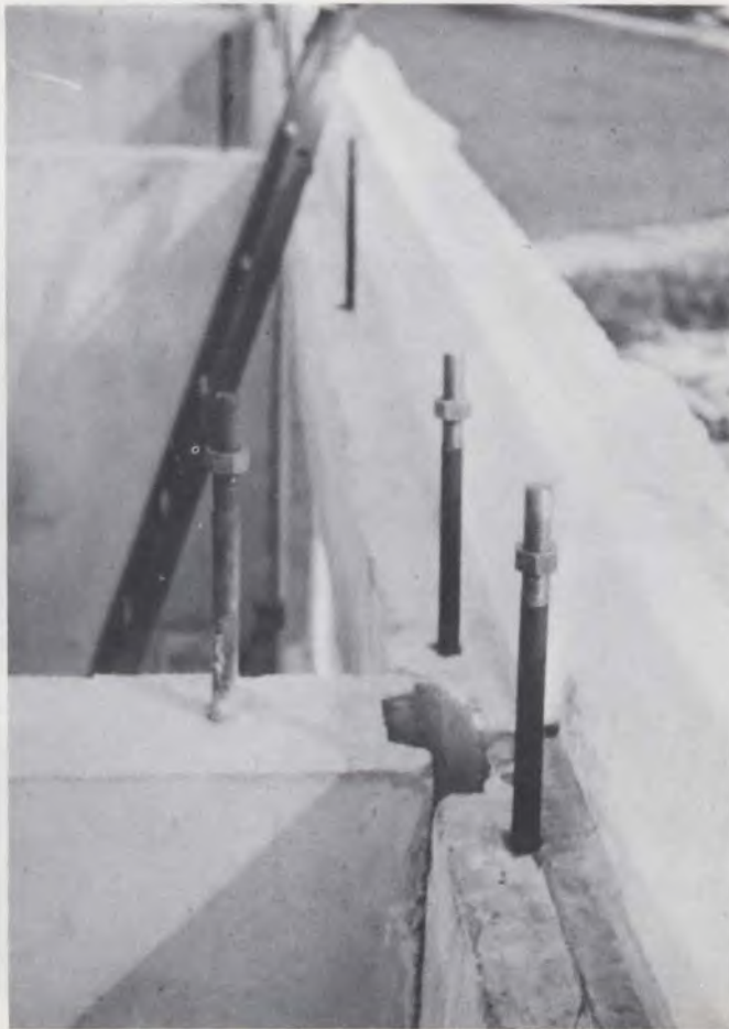
Apartment project near Malmö - showing joint of partition wall element and façade elements.
