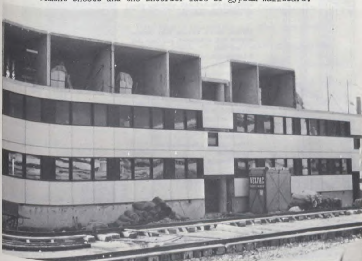
Apartment building under construction. Material to finish interior of apartments is stored inside building prior to erecting the façades.
