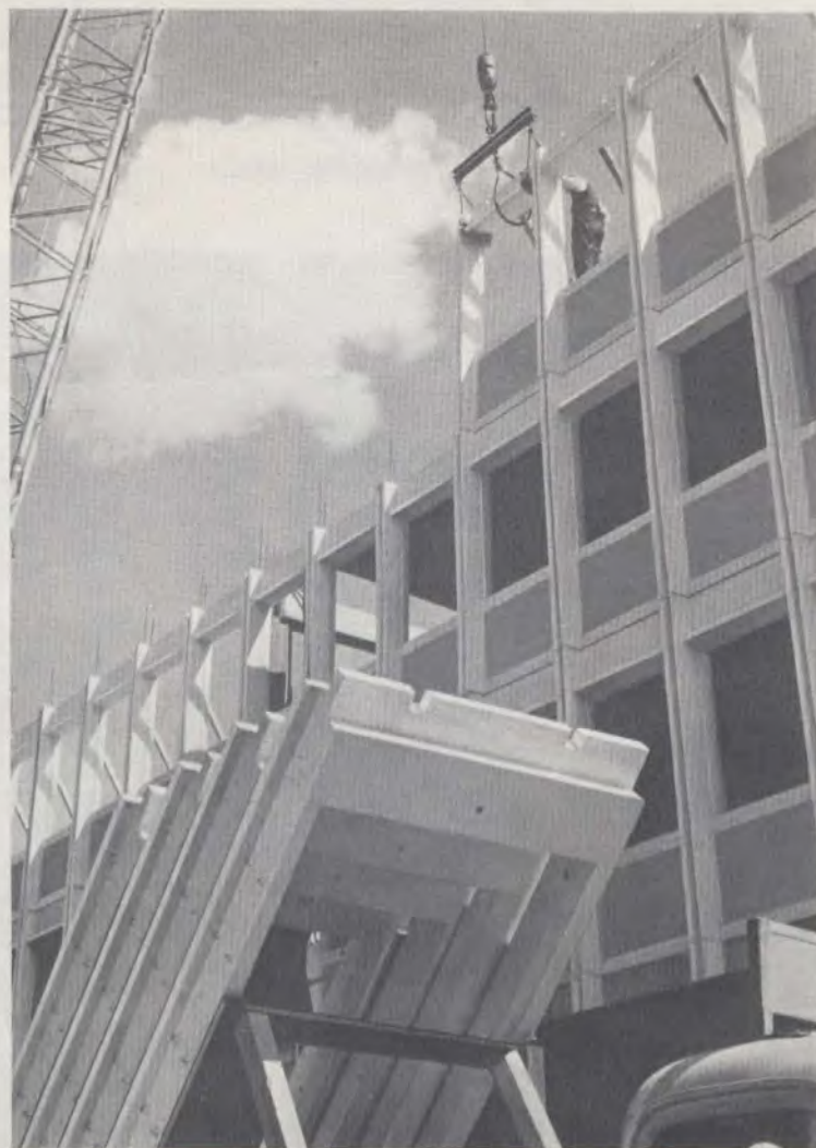
Laingwall unit lifted by crane from lorry direct into final position. Precast floors provide working platform.
