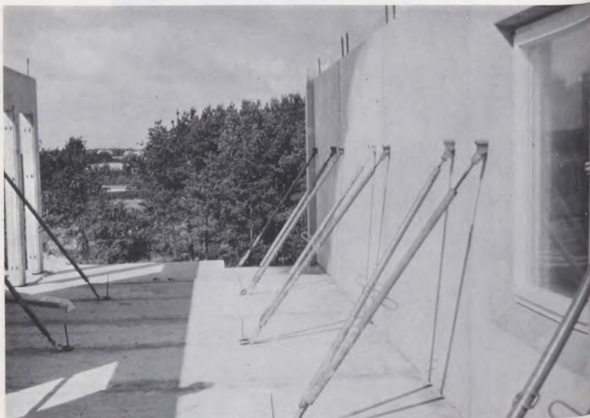
Apartment project near Malmö - showing wall elements held in position by inclined props.
