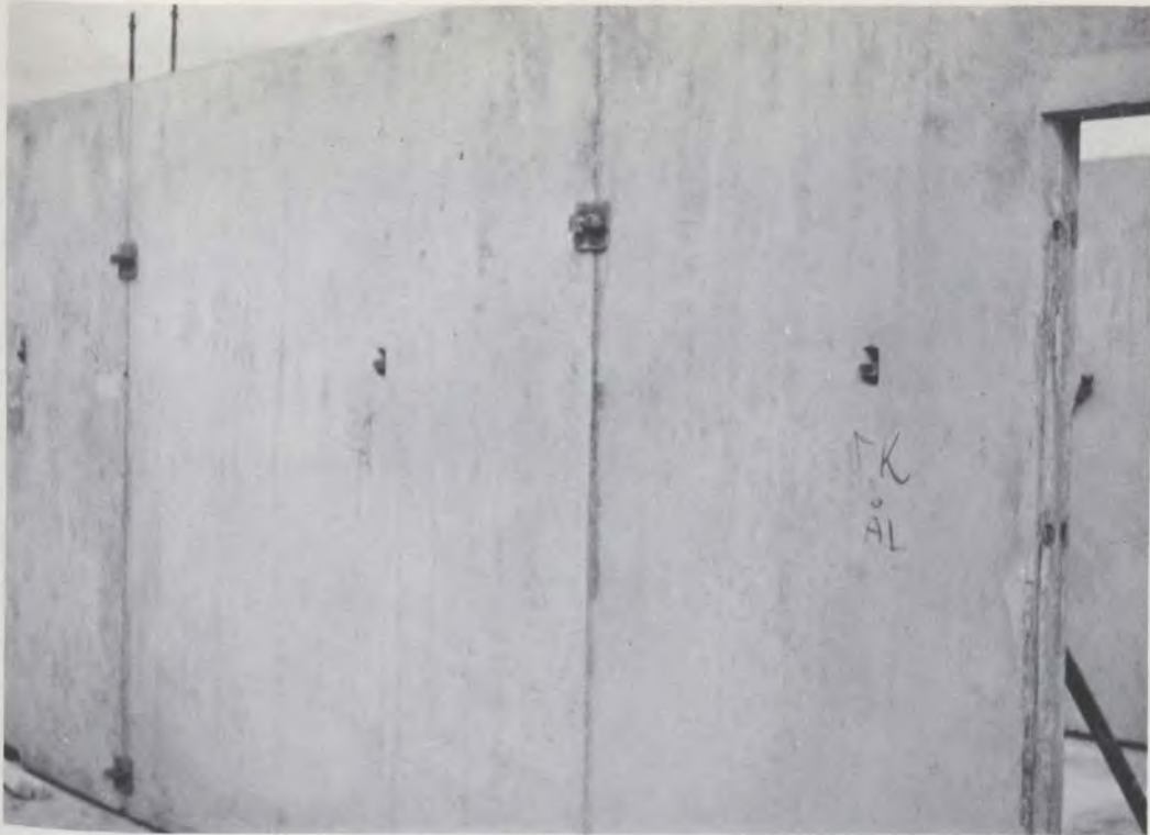
Apartment project near Malmö - showing how props are temporarily fastened to wall.
