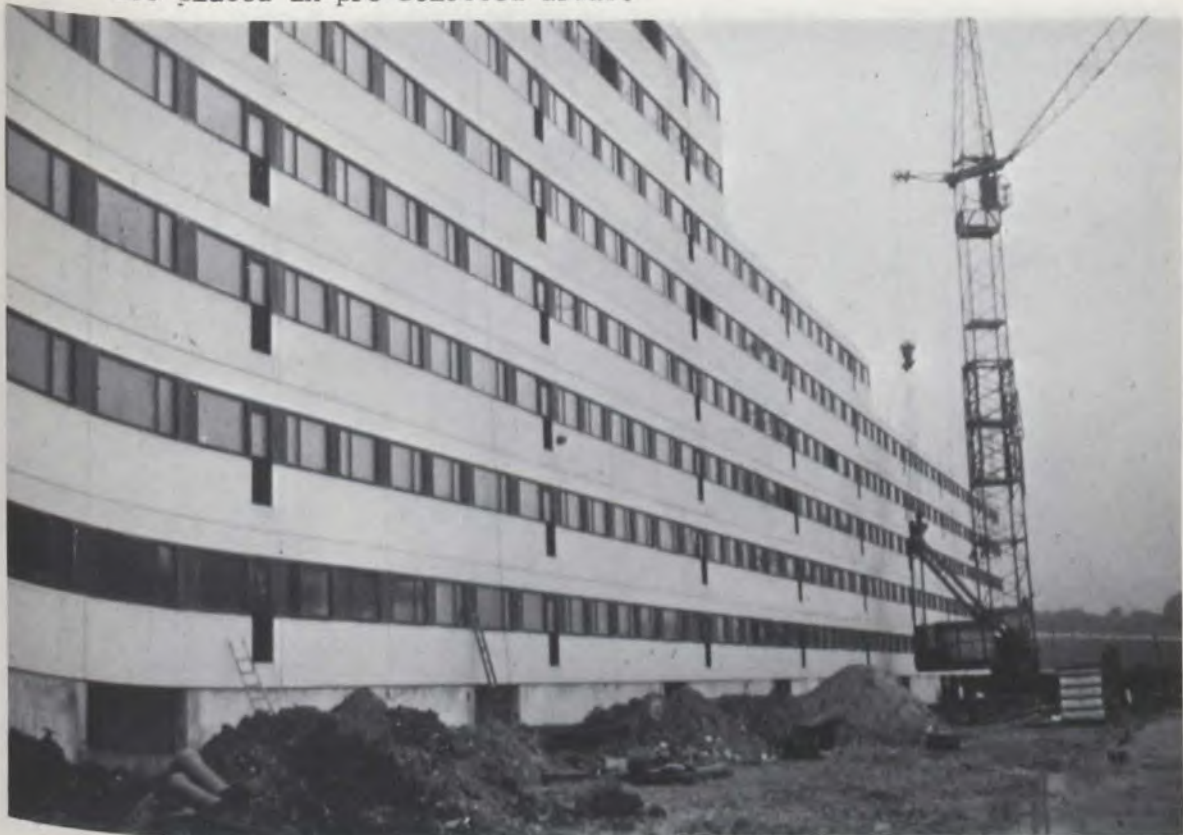
Low rent apartment building near Copenhagen. Room size façade panels are of prefabricated wood elements covered with asbestos cement sheet on the outside and gypsum wall board on the inside.
