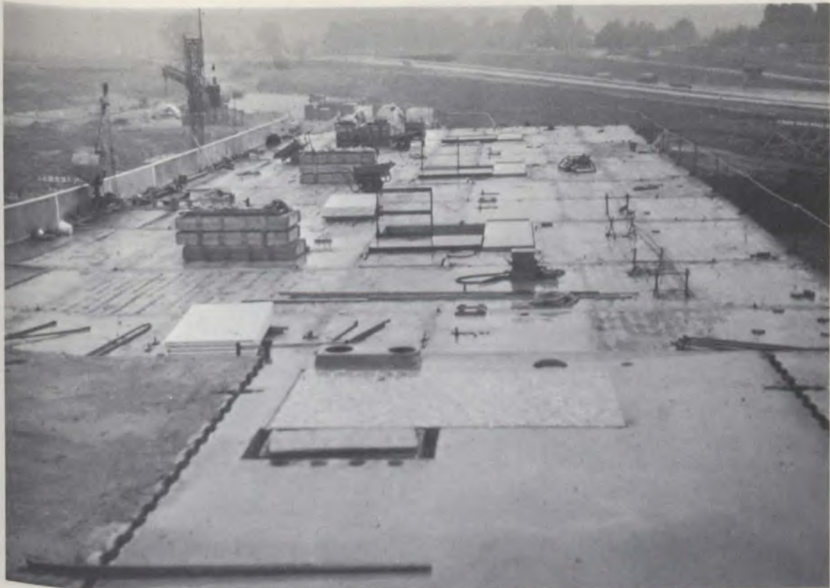
Construction site near Copenhagen showing assembled floor ready to receive wall elements. All fittings and equipment are placed in pre-selected areas.
