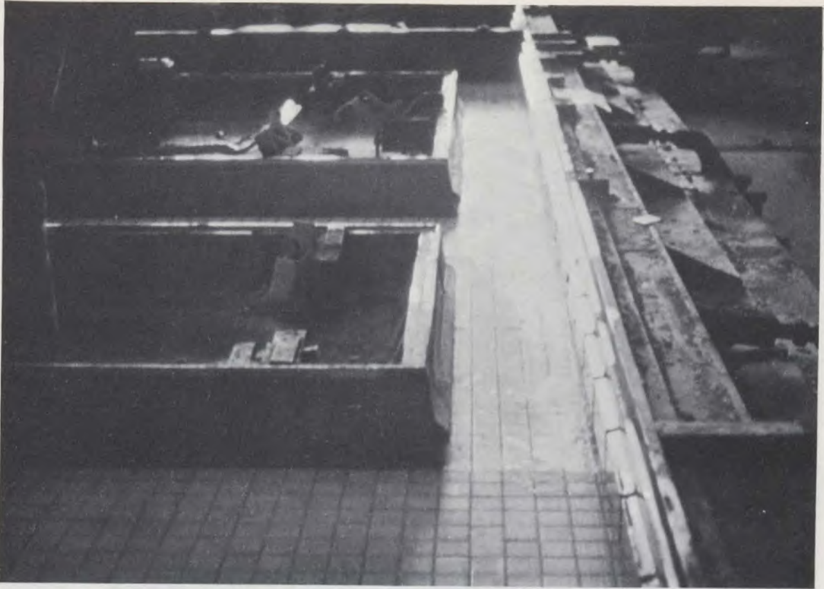
Casting table showing window opening and ceramic tiles applied on the face of the mould.
