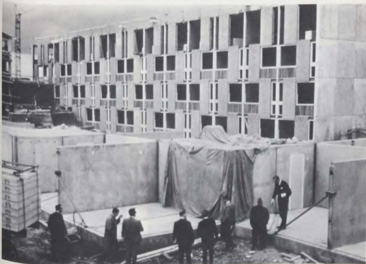
Corpus unit installed.
