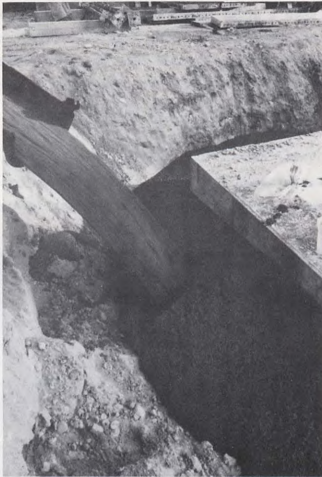
Figure 6: Placing Controlled-density Fill during the Construction of Foundations. (Courtesy of Ontario Hydro)
