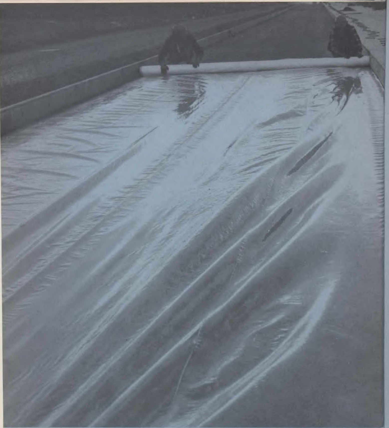
Polyethylene film is now used in building modern highways. The film is used as a barrier to keep moisture in the concrete from seeping into the ground.
