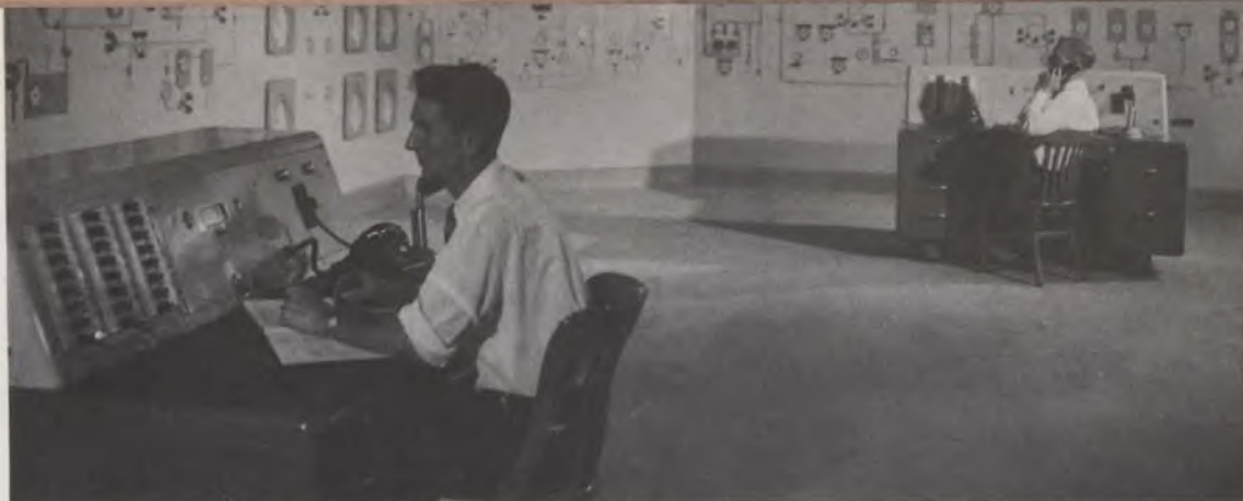
One of the two control rooms at the nylon intermediates plant of Du Pont of Canada Ltd. at Maitland, Ontario. Since 1953, several expansions have enabled it to keep up with the growing demand.
