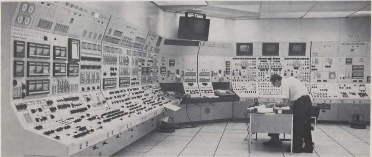
Control room at a Canadian nuclear power station.
