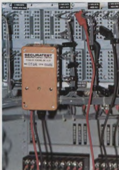
Continuity testing in live circuits can be made with this device from Securatest Manufacturing Ltd.
