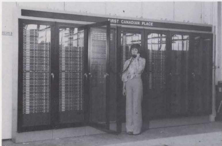
High-rise buildings present a particular challenge to fire protection systems because of their height, large floor area and high population density. Reliable communications are vital during a fire emergency and complete electronic supervision has proved to be the essential key.
