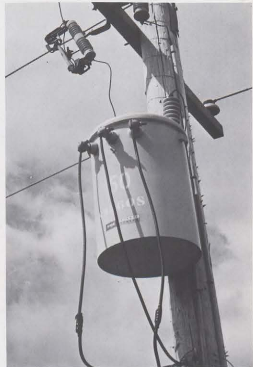
Canadian overhead distribution in residential areas employs single-phase transformers and associated protective equipment.
