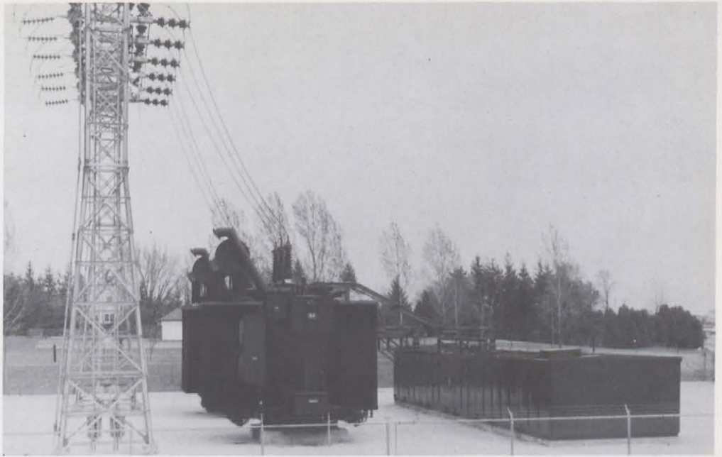
Typical sub-transmission distribution station showing structure, transformer and outdoor switchgear.
