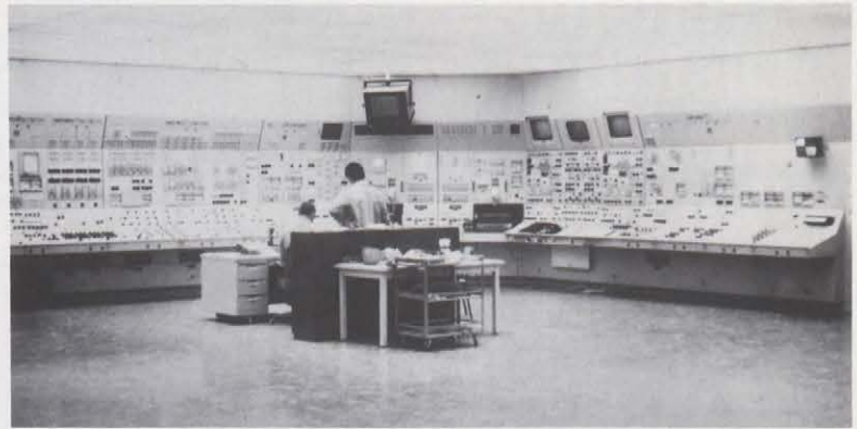
One of the four nuclear reactor/turbine panels controlling a 500 MW generating unit at the Pickering station.
