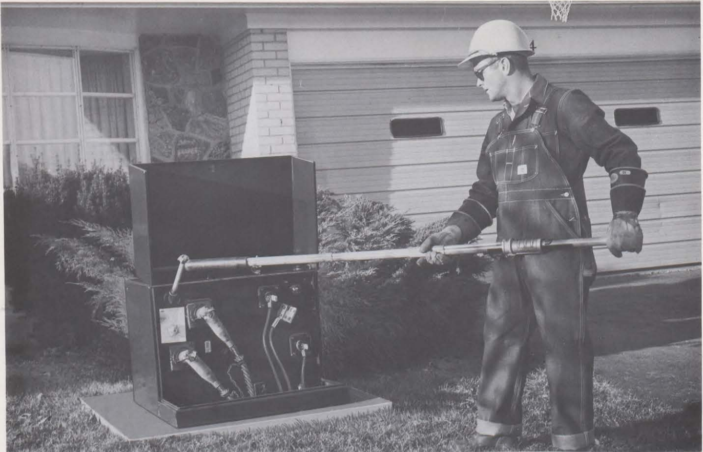
Canadian underground distribution in residential areas uses transformers and associated switching mounted on concrete pads.
