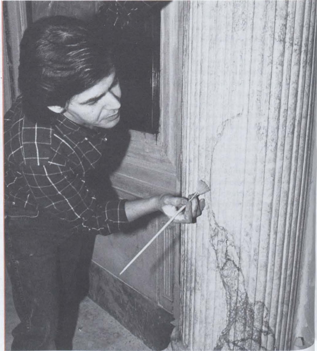
The federal government contributed $5 million to the renovations of the Elgin and Winter Garden Theatre complex. Shown here is restoration consultant, David Hannivan, applying false marble to lobby column. (Photo courtesy of the Elgin and Winter Garden Project)
