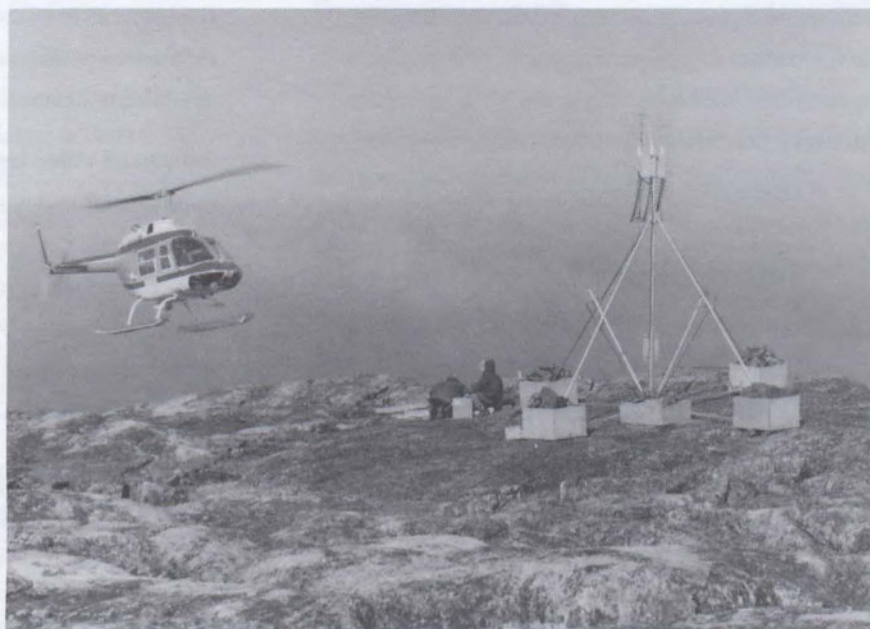
Technicians test a UHF antenna installation in Northern Canada.
