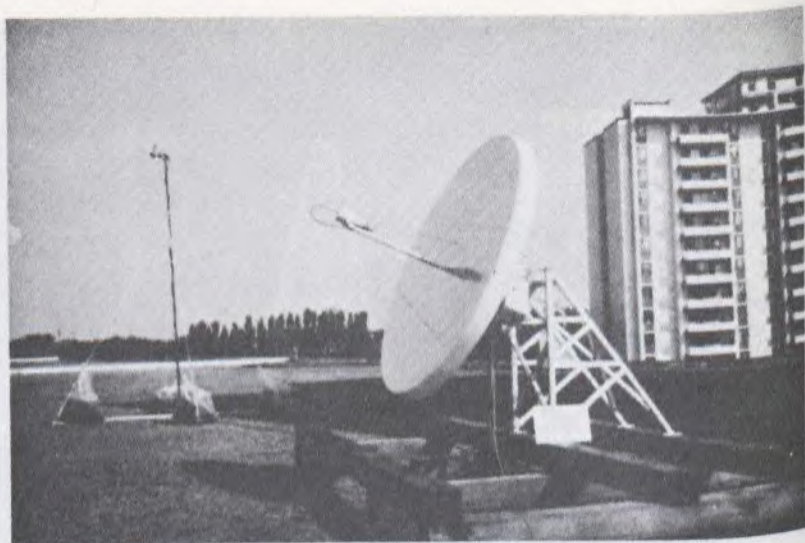
1.6 METER ANTENNA (Community Reception) Motorized mount, Engineering Headquarters, Montreal
