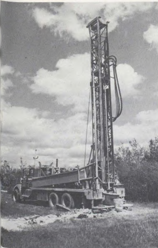
Many modern farm water and sewage systems were installed under the farm water service program.
