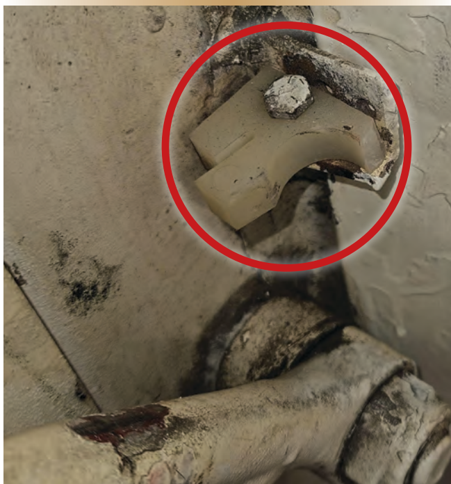
Figure 4. Broken door holdback. The right-hand side of the holdback notch has broken away, preventing the door handle from being secured.
