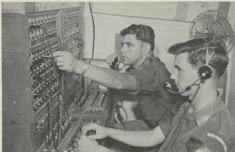
A field switchboard at Rafah Camp.
