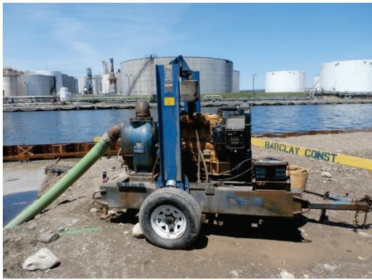
Pump used to discharge brown water into Hamilton Harbour (Lake Ontario)
