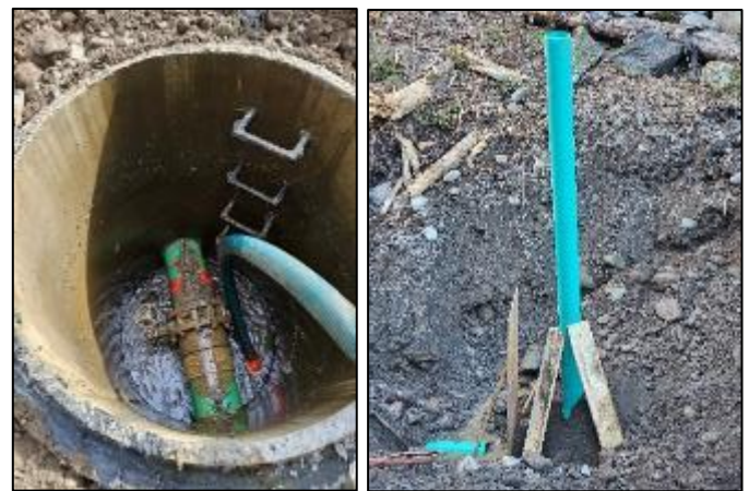
Figure 1. Partially excavated flooded manhole with broken valve (left). Buried replacement valve with new access pipe (right).
