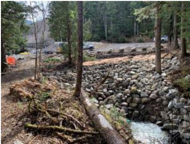
Figure 2. View of rip rap wall, exit pipe and valve access pipe.
