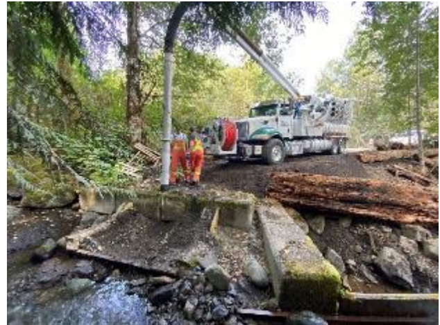
Figure 1. Maintenance for the existing intake using a vacuum truck to remove accumulated bedload.
