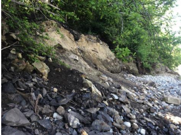
Reach 2 erosion at RDN trail head
