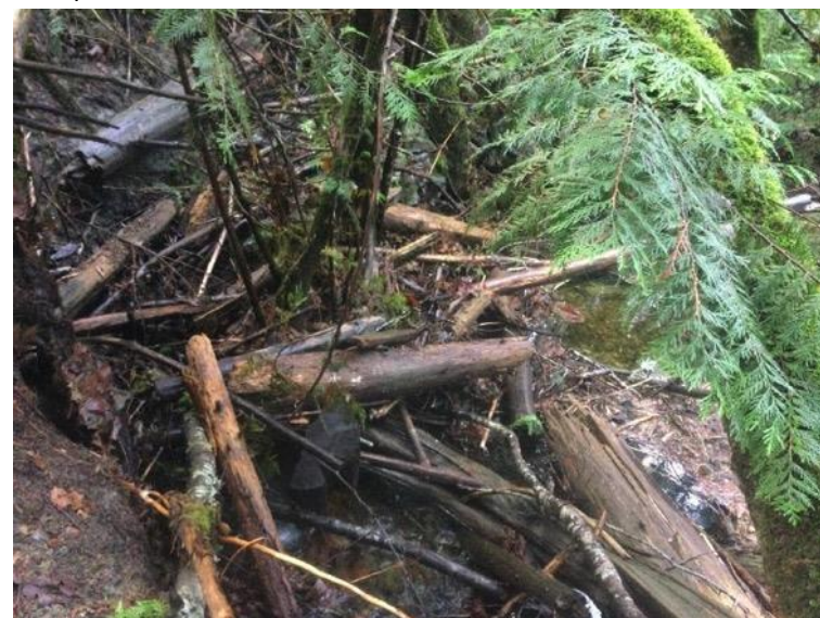
4.) R13 – Wolf Creek plugged culvert
