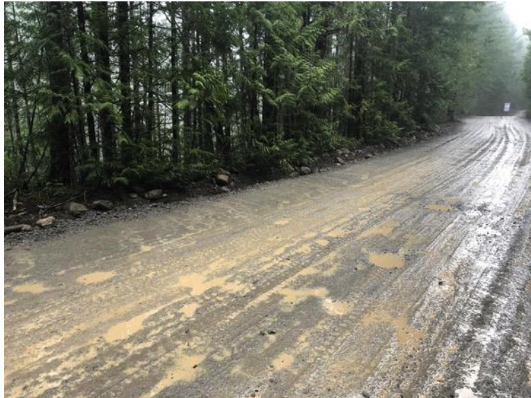
3.) Road is 10m from river, note grader berm on river side
