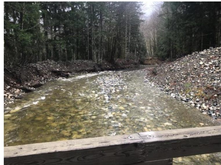
4.) R18 – Dash Creek sediment deposits at road crossing
