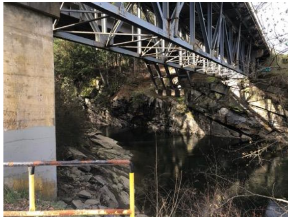
Hwy 1 Bridge drain pipes go direct to pool.
