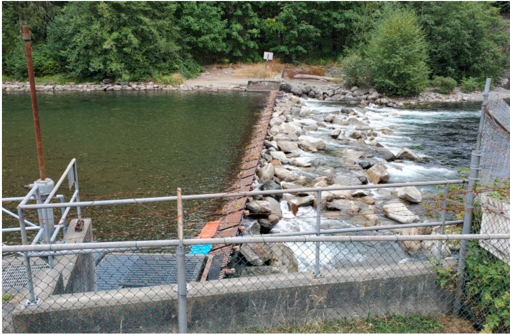
Figure 62. Puntledge hatchery fence after cleaning gravel/debris. Flow passes through rather than over fence (Photo DFO hatchery staff).
