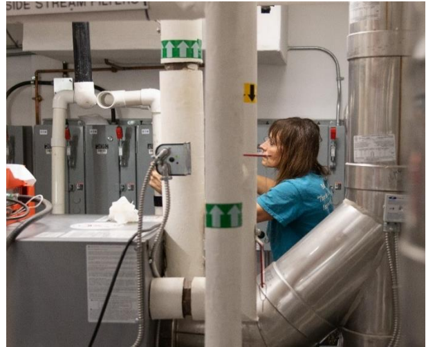
Photo 9: Commissioning the Bioelectrochemical Anaerobic Sewage Treatment System in a Triplex at Canadian High Arctic Research Station Photo: Polar Knowledge Canada
