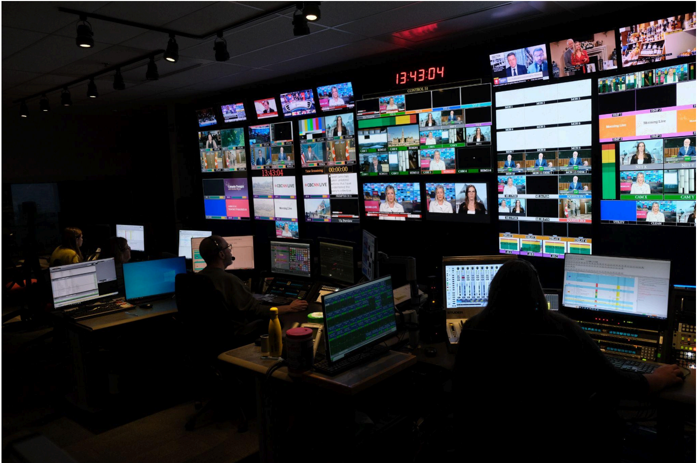
The Toronto Broadcast Centre (TBC) control room
