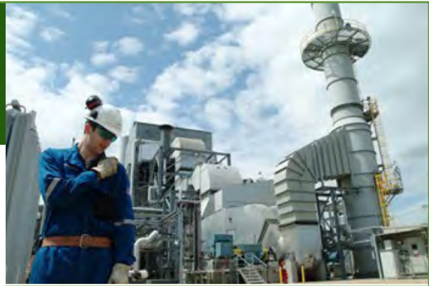
Air Products hydrogen production facility near Edmonton, AB.
