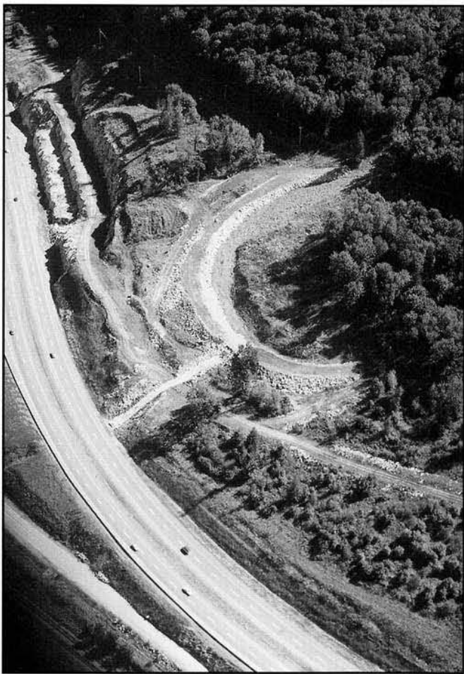
Figure 41. Debris deflection barrier (or berm) constructed to protect Trans-Canada Highway and Canadian National Railway rail track, 5 km southwest of Laidlaw in the Fraser Valley. GSC 1994-492E
