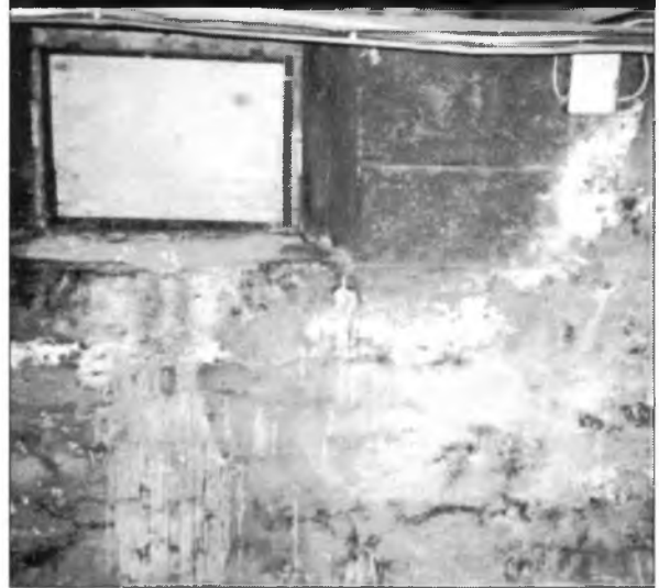
Efflorescence and evidence of water leaks around boarded-up window in basement Buchan, Lawton, Parent Ltd
