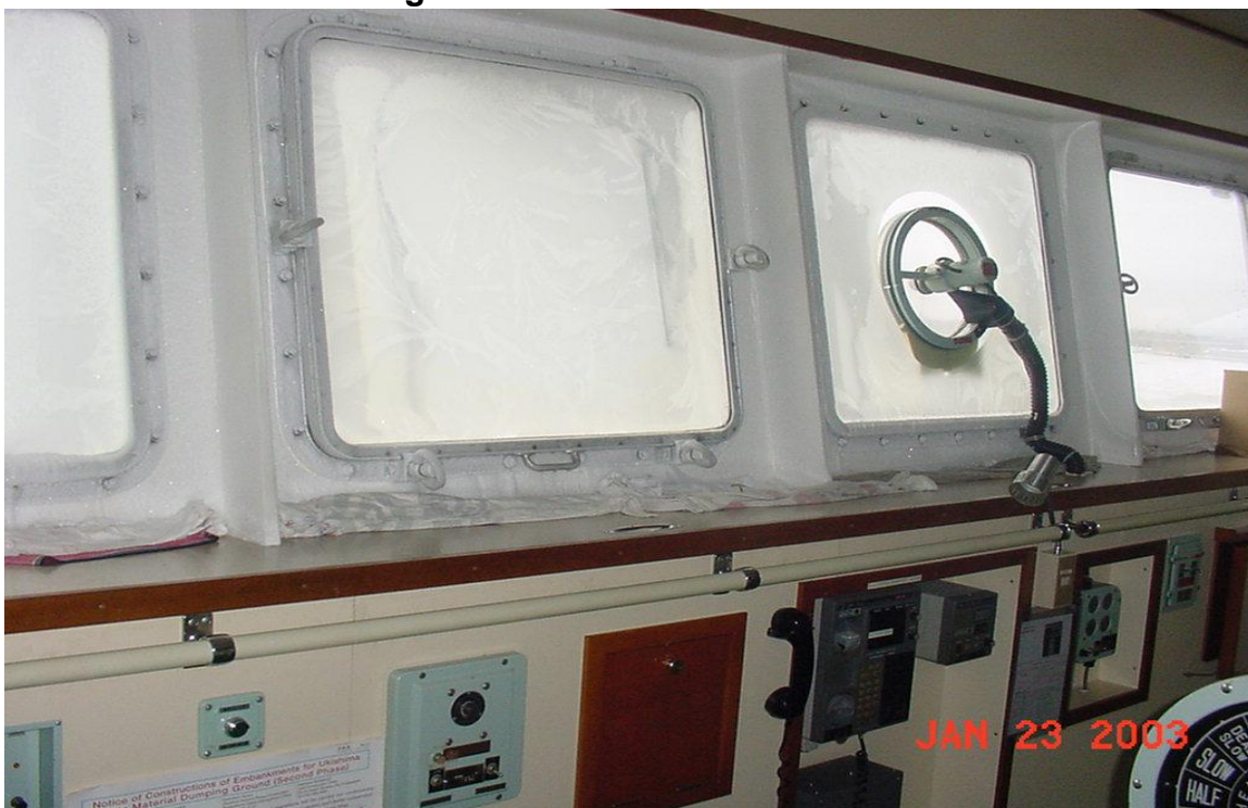
Figures 9.1B – Deficient wheelhouse heating combined with a high rate of humidity
