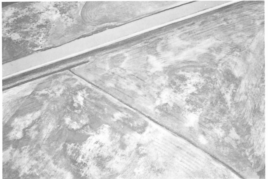
FIG. 5 Damage caused by seepage from canal.
