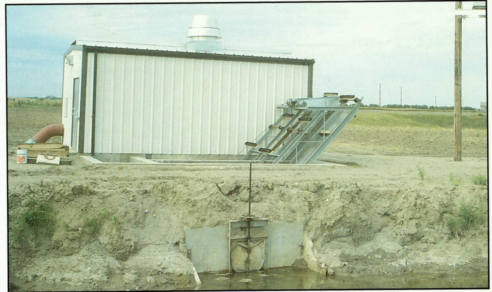
Pump site beside the main canal for the South Saskatchewan River Irrigation District #1 showing intake and scrubbers. The scrubbers remove algae and debris from the intake screen.
